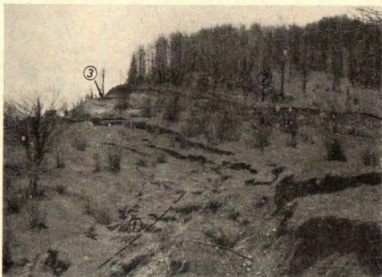
Sl. 3. Glavna pukotina prema cesti — Main fissures view toward the road — 1 glavna pukotina — main fissure — 2 uvala stare usjekline — old depression — 3 usjek nove ceste — new road cut
