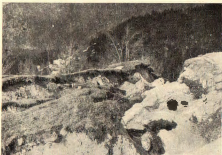
Sl. 2. Pukotine uz cestu 6827 — Fissures along the road
