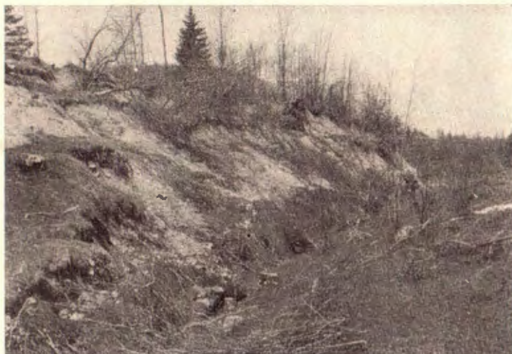
Sl. 4. Glavna pukotina prema pruzi 78 — Main fissure, view toward the railway
